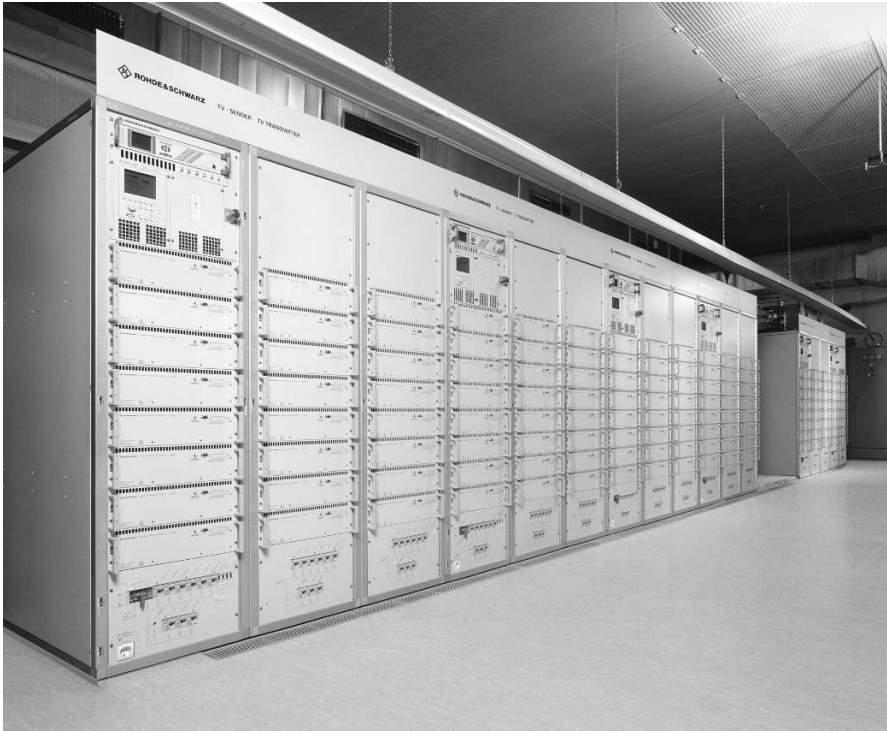
Fig. 31.17. DVB-T transmitters Olympic Tower Munich; manufacturers photo, Rohde&Schwarz.
