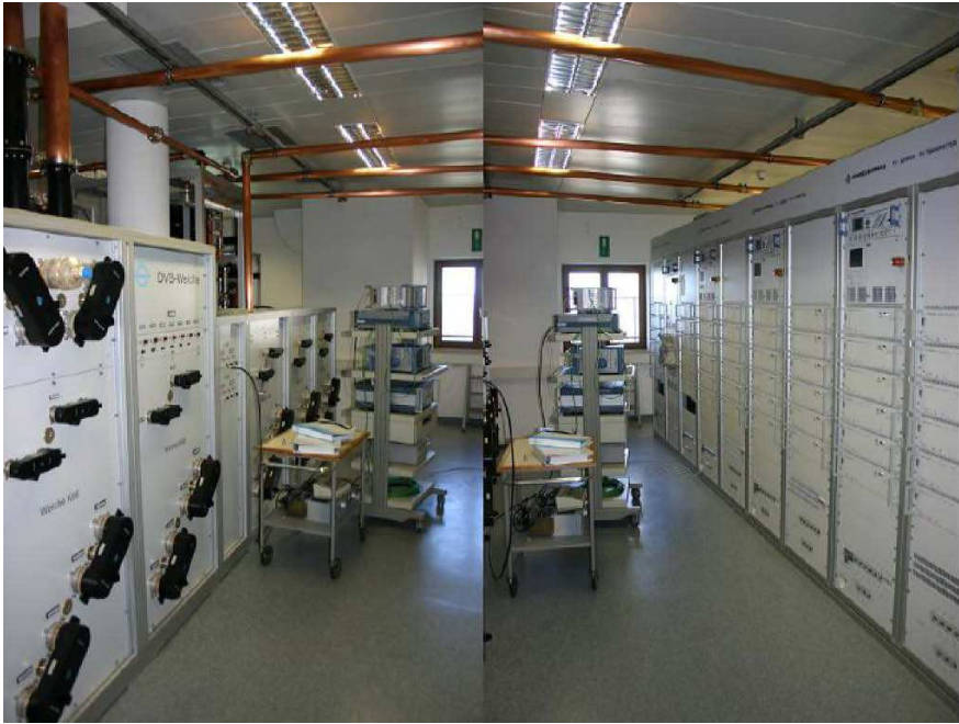
Fig. 31.14. Wendelstein transmitter hall; antenna combiner (left) and UHF transmitters (right)
