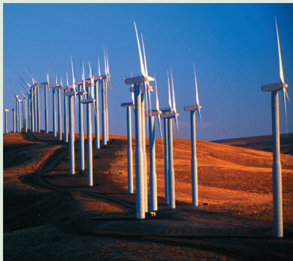
Stateline Wind Generating Project in Walla Walla, Washington.
