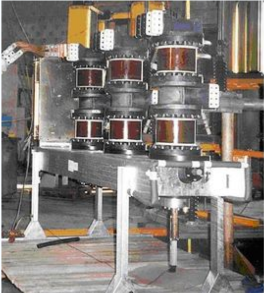
Generator circuit breaker rated for 17.5 kV and 63 kA
