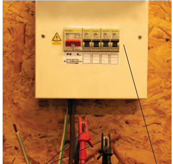
Connected to live conductors
