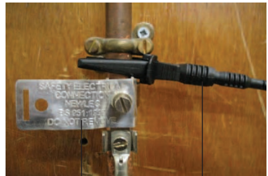
Banded metalwork Other end of test lead
