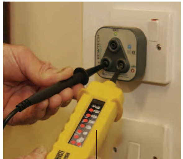
No voltage lights lit
