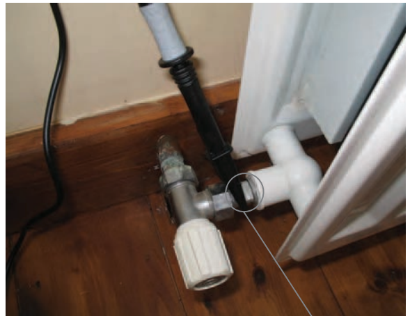
Unpainted metal work
