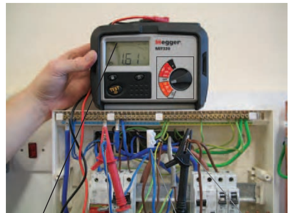
Resistance double that of phase conductor P2 P1 joined to N2 N1
