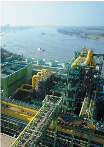
Figure 13.14: Coke oven plant in Duisburg-Schwelgern. © Thyssen-Krupp
