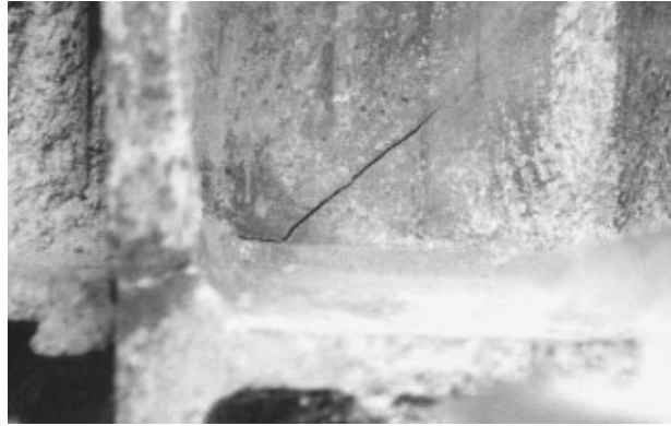
FIGURE 9.11 Photograph of crack through the column flange and into the column web or panel zone of connection.
