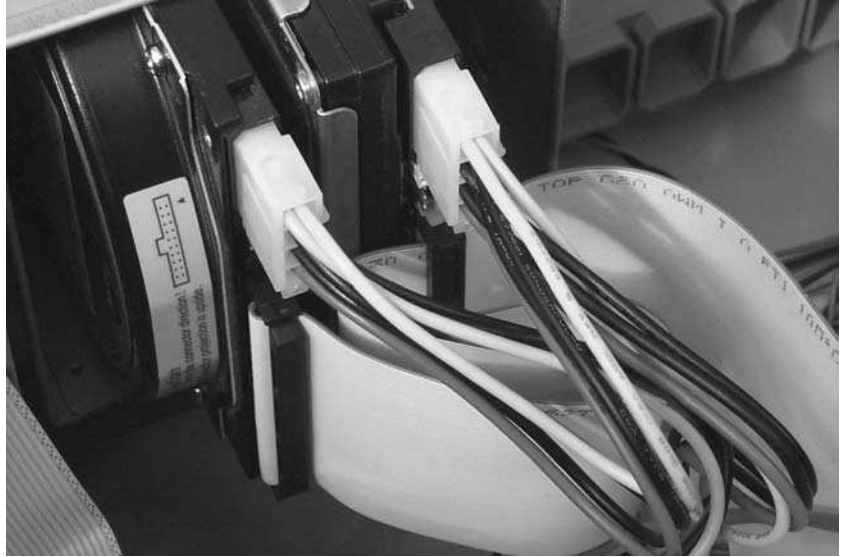
Photo 1.16 Power and data connectors at the rear of two hard drives
