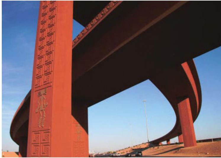
Exhibit 1.18 The interchange between the Red Mountain Freeway (202) and U.S. 60 in Mesa, Arizona, is a good example of using Southwest-type texture and color to produce a beautiful blend of tall piers and gracefully curved girders. (Photo courtesy of Arizona DOT.)
