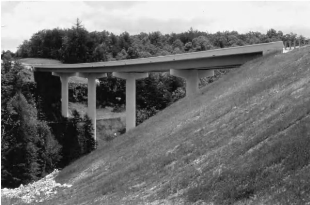
Fig. 3.8 Example of superstructure continuity on single hammerhead piers. (Photo courtesy of Tennessee DOT—Geo. Hornal, photographer.)
