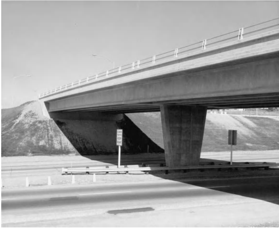
Fig. 3.32 Prestressed girders frame into the side of the supporting pier, eliminating from view the usual cap beam. (Permission granted by the California DOT.)
