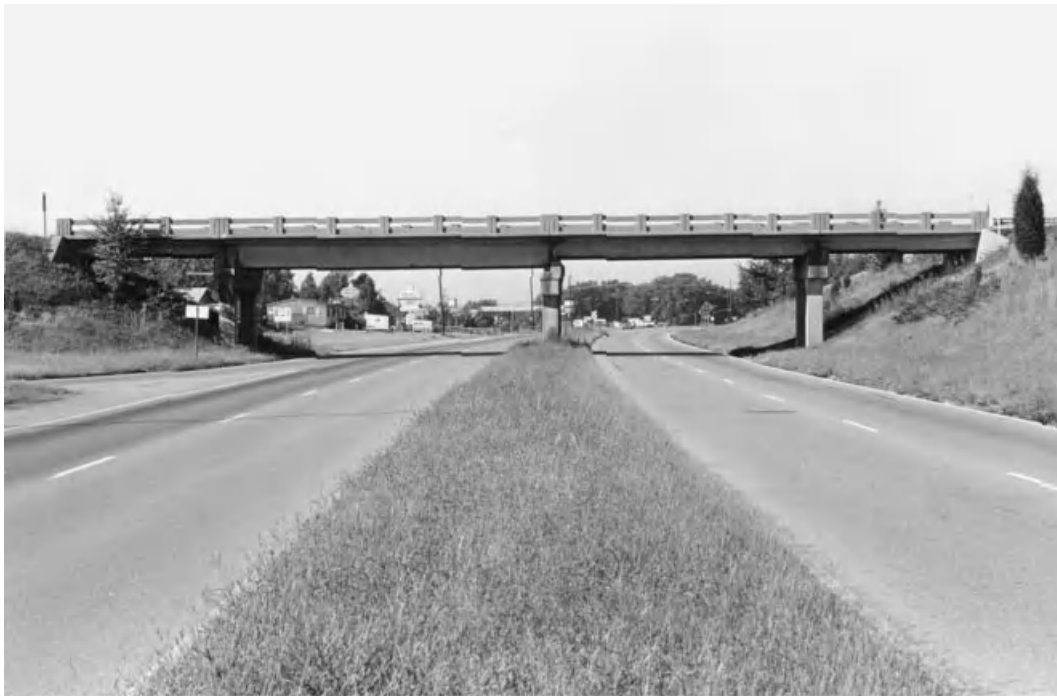
Fig. 3.9 Example of poor depth transitions and awkward configurations due to lack of superstructure continuity. (Photo courtesy of Tennessee DOT.)
