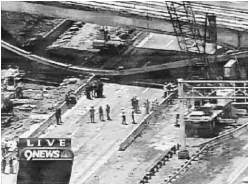
Fig. 2.18 Bridge failure near Golden, Colorado. (Photo from Golden Fire Department Annual Report 2004, Golden, Colorado. http://ci.golden.co.us/files/2004fdreport.pdf .)
