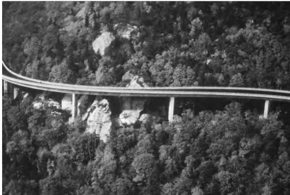
Fig. 3.16 Blue Ridge Parkway (Linn Cove) Viaduct, Grandfather Mountain, North Carolina (Gottemoeller, 1991). (From Bridge Aesthetics Around the World , copyright © 1991 by the Transportation Research Board, National Research Council, Washington, DC. Reprinted with permission.)
