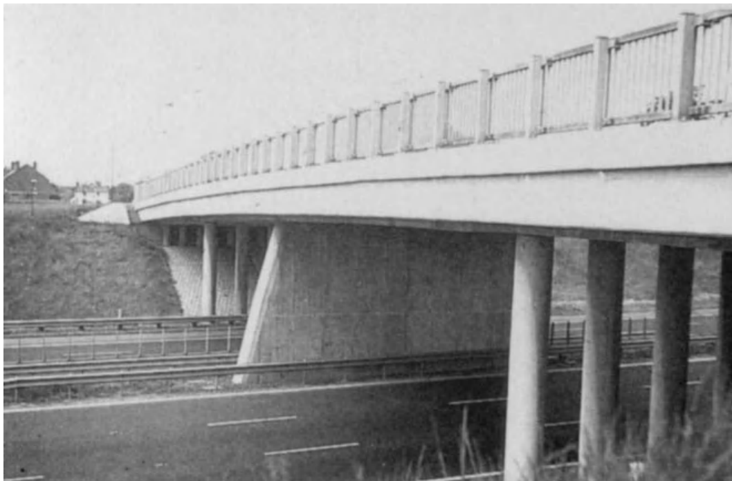
Fig. 3.37 Bridge with displeasing mixture of supports (Murray, 1991). (From Bridge Aesthetics around the World , copyright © 1991 by the Transportation Research Board, National Research Council, Washington, DC. Reprinted with permission.)
