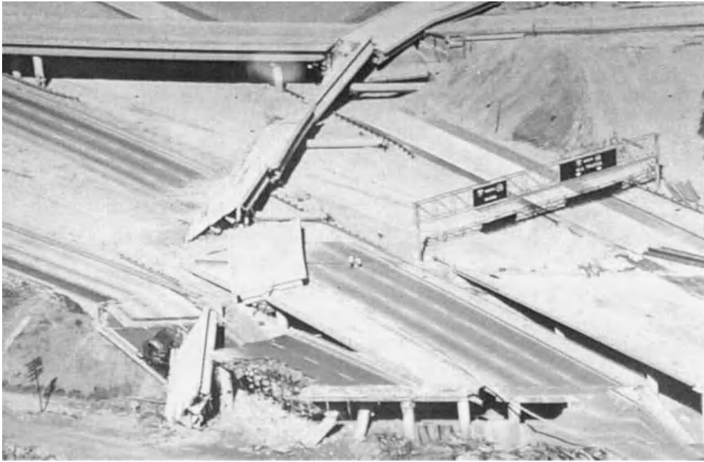
Fig. 2.4 View looking north at the I-5 and I-210 interchange after the quake showing the collapsed South Connector Overcrossing structure (bridge 2) in the center, the North Connector Overcrossing structure (bridge 3) at the top, and bridge group 4 at the bottom. (Photo courtesy E. V. Leyendecker, U.S. Geological Survey.)
