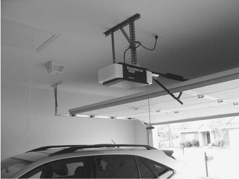
This small electric motor opens and closes a garage door. (Kyle Kirkland)
