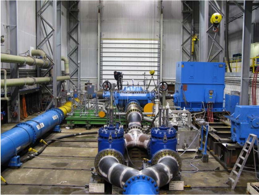
Figure 3.7 One of four test beds at Sulzer Pumps' UK facility
