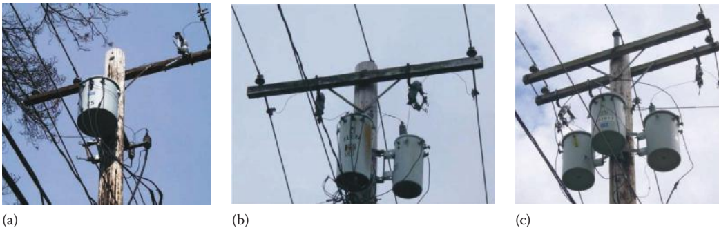
FIGURE 11.15 Transformer banks: (a) single-phase transformer, (b) two transformer bank, and (c) three transformer bank.
