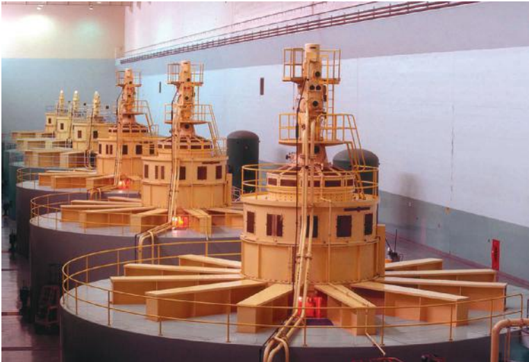
FIGURE 4.5 Hydroelectric turbine-generator units at the lower granite power plant, Walla Walla, Washington. (Image courtesy of U.S. Army Corps of Engineers, Louisville, KY.)
