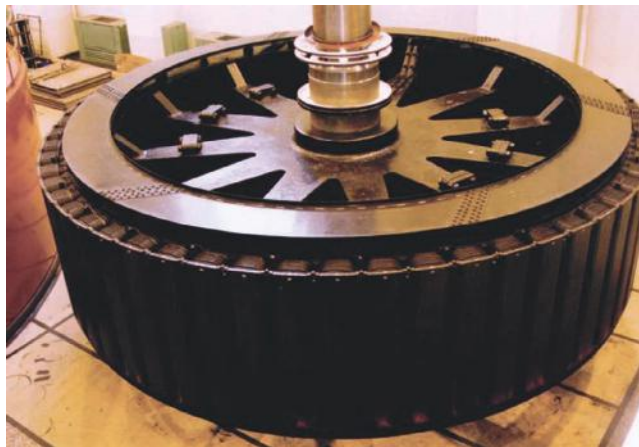
FIGURE 12.34 Rotor of a synchronous generator in Grand Coulee Dam. (Courtesy of the U.S. Bureau of Reclamation, Washington, DC.)
