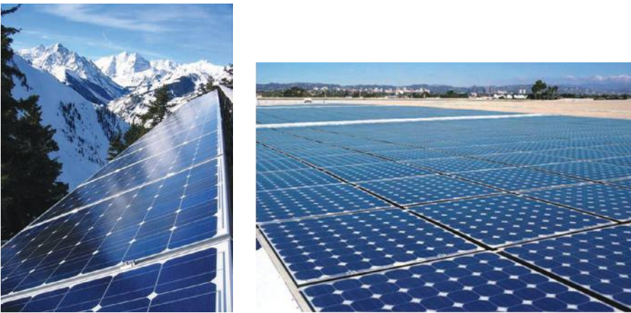
FIGURE 6.37 High power PV systems. (Images are courtesy of the US Department of Energy, Washington, DC.)
