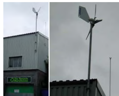
Figure B.9. An Ampair “600 W” micro-turbine. The average power generated by this micro-turbine in Leamington Spa is 0.037 kWh per day (1.5 W).
