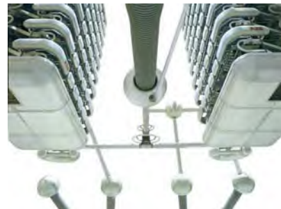
Figure 25.13. A high-voltage DC power system in China. Photo: ABB.
