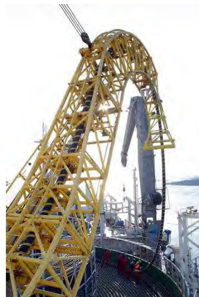
Figure 25.7. Laying a high-voltage DC link between Finland and Estonia. A pair of these cables transmit a power of 350 MW. Photo: ABB.
