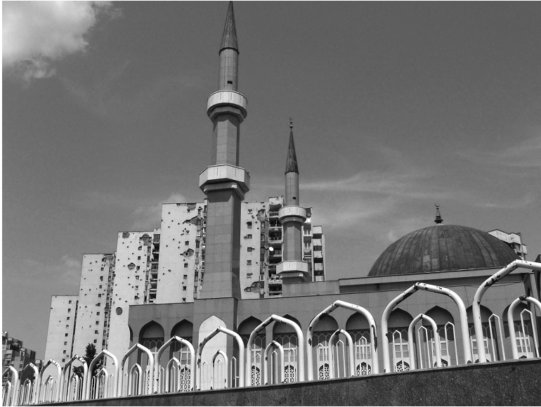
Fig. 15 Mortar damage in Sarajevo (by Richard Mills)
