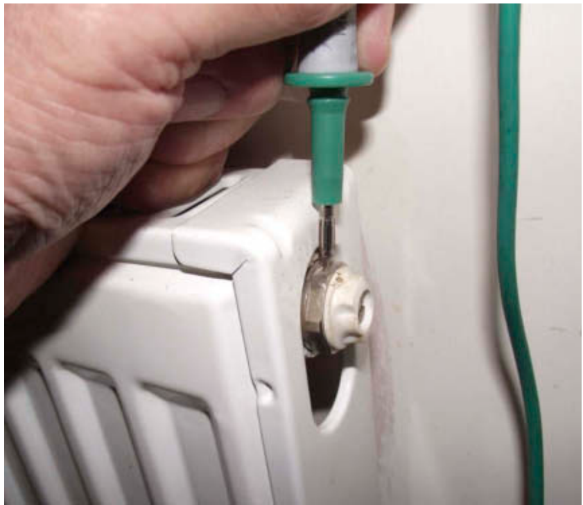
Figure 4.22 Lead on unpainted part of radiator
