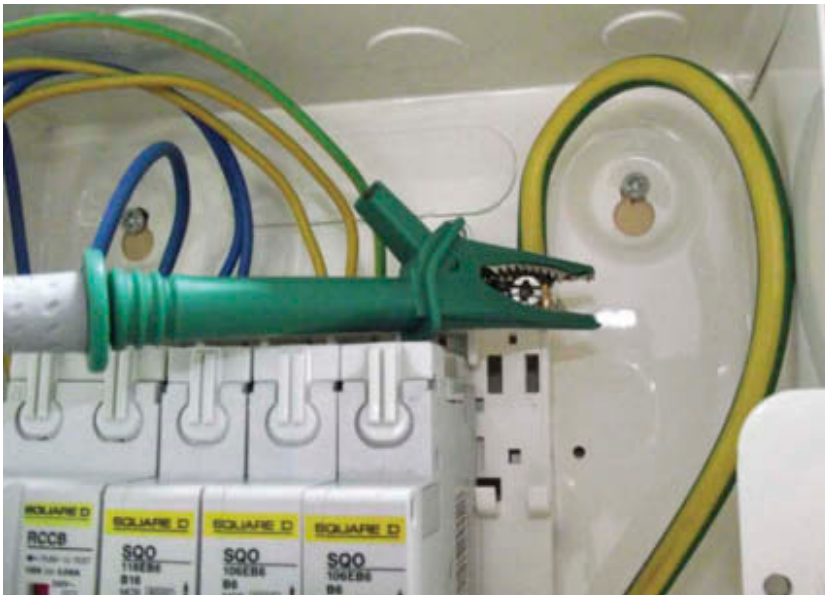
Figure 4.27 Lead connected to earthing terminal
