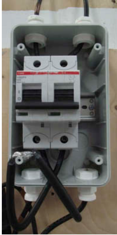
Figure 10.13 D.C. cables linked
