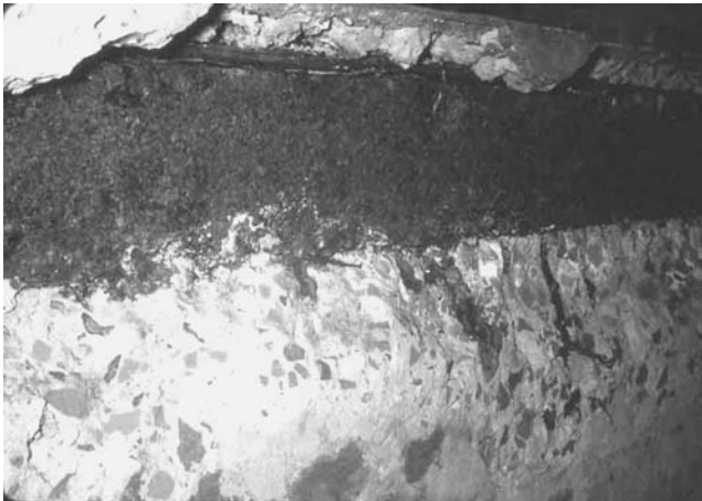
Figure 2.5 Corrosion of reinforcing bars at Alcatraz Prison, California, due to use of aggregates contaminated with sea salts.
