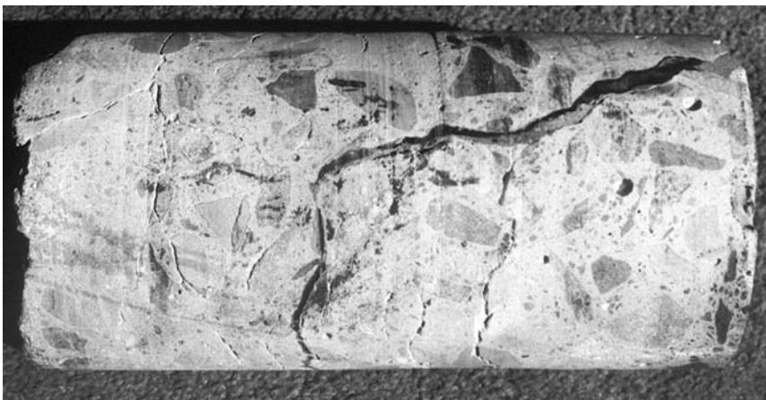
Figure 6.12 Cracking of core due to internal ASR and external drying.
