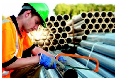
▲ PVC pipe is widely used in industry.
