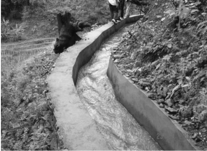
FIGURE 5.2 A typical cement masonry-lined headrace canal in a micro hydropower plant.
