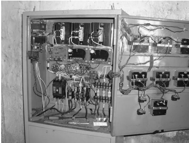
FIGURE 2.30 Control panel of a micro hydropower plant combined with the ELC.
