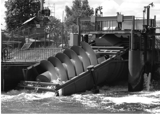
FIGURE 12.6 Archimedes screw turbine in use in Poland (diameter 3 m; flow of 6 m 3 /s; height 1.8 m; maximum power 80 kW). (Courtesy of Pesymista [own work], CCBY-SA 3.0, https://commons.wikimedia.org/wiki/File:Turbina_Archimedeses_MEW_Goryn.jpg#filelinks .)
