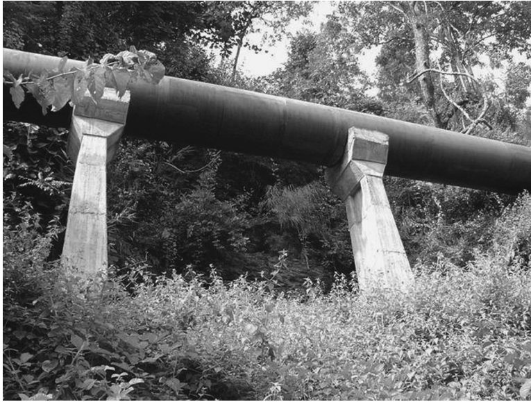
FIGURE 2.15 A penstock crossing for a 3-MW hydropower plant, Nepal.
