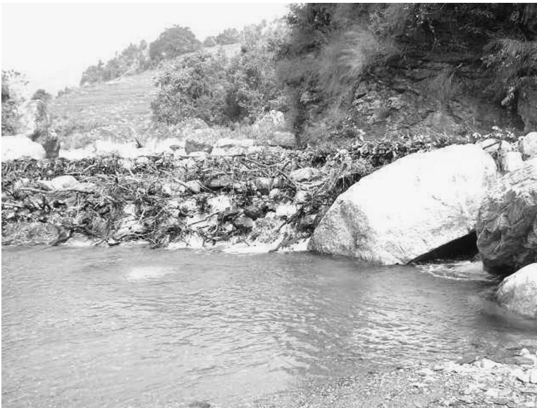
FIGURE 4.6 A temporary weir built from boulders and brushwood to divert water into the intake of a micro hydroelectric power plant, Nepal.
