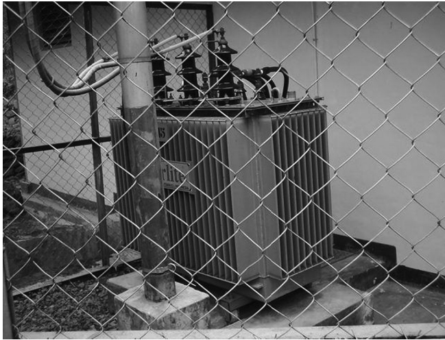
FIGURE 2.32 An outdoor transformer for a micro hydropower plant, Indonesia.
