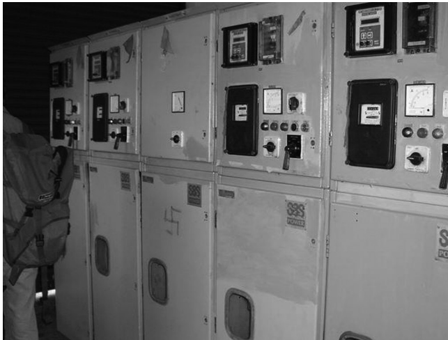
FIGURE 2.31 Control panel for a mini hydropower plant.
