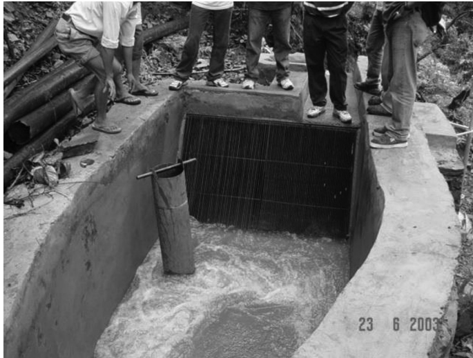
FIGURE 2.17 A typical forebay installed in a micro hydropower plant, Nepal.
