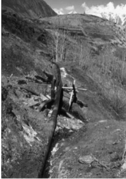
FIGURE 5.7 A HDPE headrace pipe used to cross steep hill slopes, Nepal.
