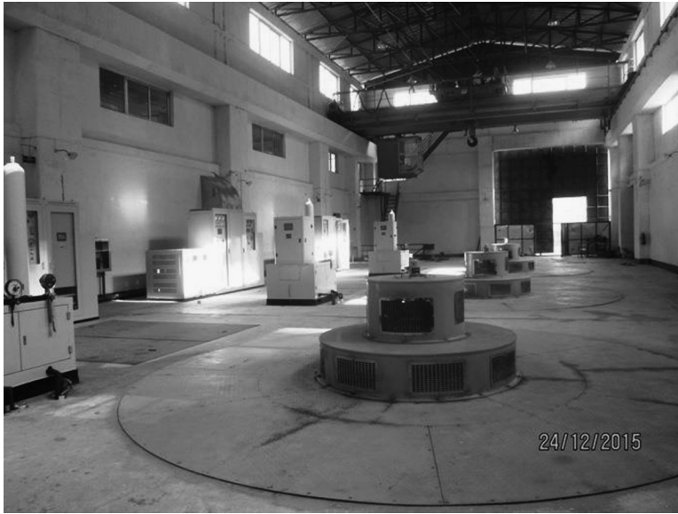
FIGURE 8.11 Generator floor level of Mai hydropower plant's powerhouse.
