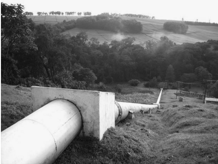
FIGURE 2.18 Penstock alignment for a 900-kW plant, Kenya.
