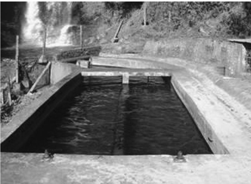
FIGURE 2.11 Combined gravel trap and settling basin of a 500 kW mini hydroelectric power plant, Nepal.
