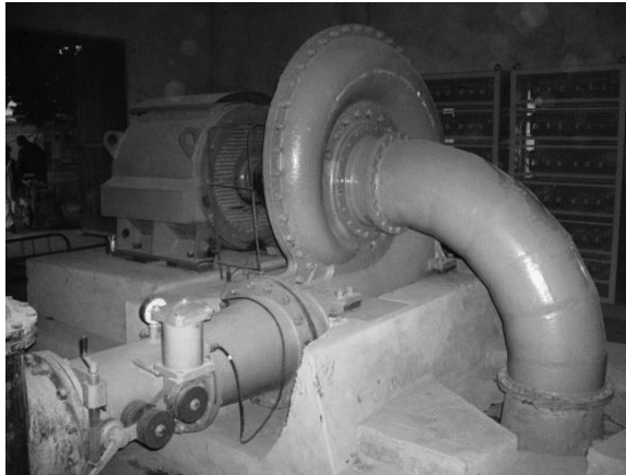
FIGURE 2.27 An induction generator coupled with a Francis turbine in a micro hydropower plant, Afghanistan.
