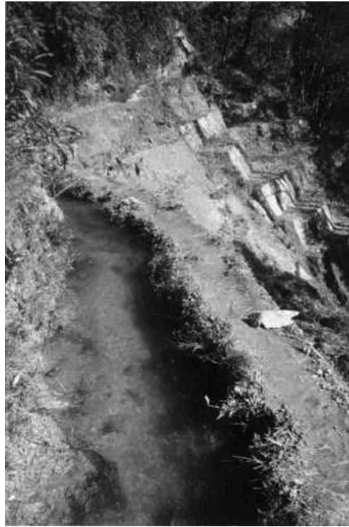
FIGURE 5.5 An unlined headrace canal used in a micro hydropower plant.
