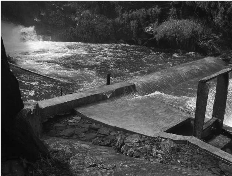
FIGURE 4.5 A frontal intake of a mini plant in the Panjshir Hydropower Plant in Nepal.
