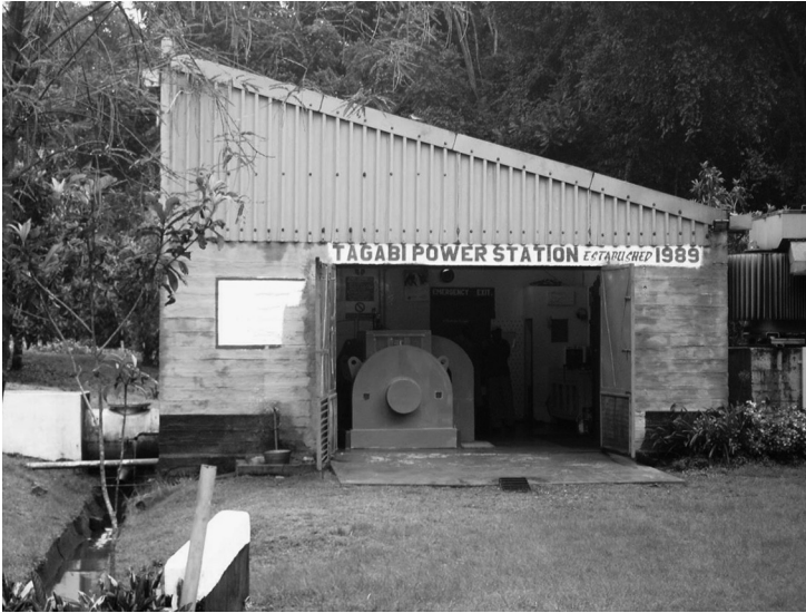
FIGURE 8.4 500-kW Tagabi micro hydro powerhouse, Kenya.
