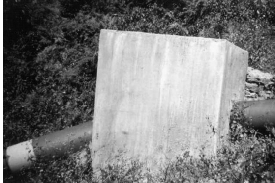
FIGURE 2.20 Reinforced concrete anchor blocks used in a mini hydropower plant, Nepal.
