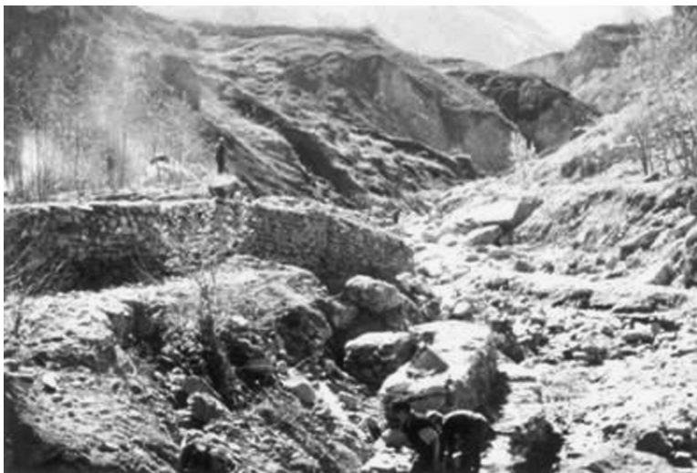
FIGURE 4.9 Partially damaged gabion weir placed across the river, Nepal.
