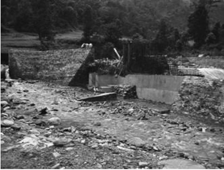
FIGURE 4.1 Flood damage at partially completed headworks structure, Nepal.
