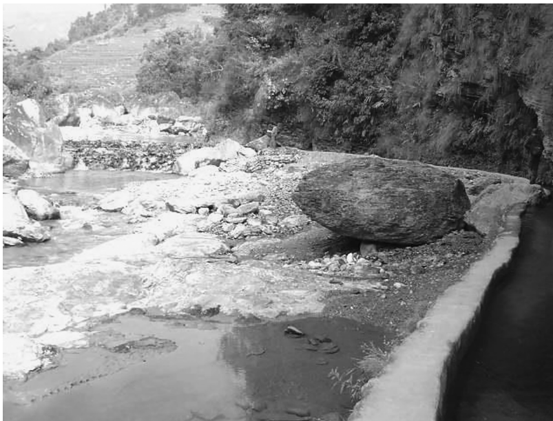
FIGURE 2.6 Typical temporary weir used in micro hydroelectric power plant.
