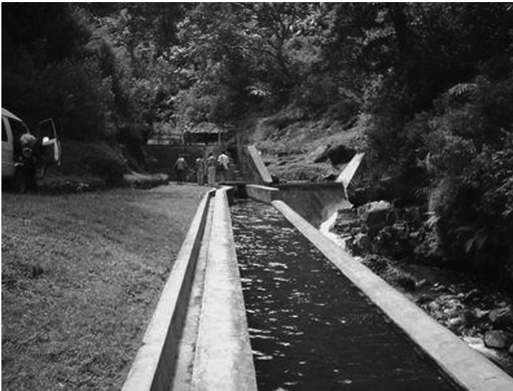
FIGURE 2.9 A reinforced concrete headrace canal used in a micro hydropower plant, Indonesia.
