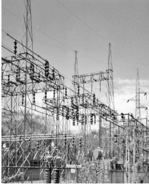
FIGURE 12.16 Switchyard protected by overhead shield wires
