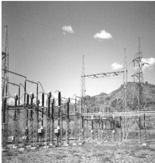
FIGURE 12.14 Switchyard using rigid bus-work
