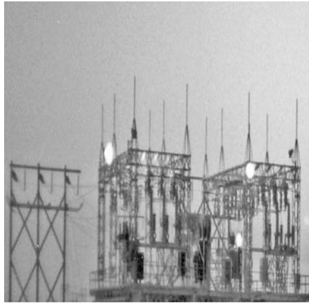
FIGURE 12.17 Switchyard protected by masts
