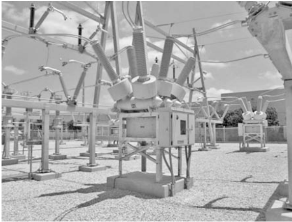
FIGURE 7.8 SF 6 gas circuit breakers
