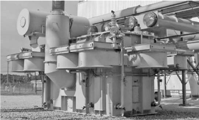
FIGURE 5.9 Generator step-up transformer
