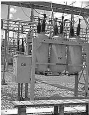
Oil Circuit in a 41 kV
