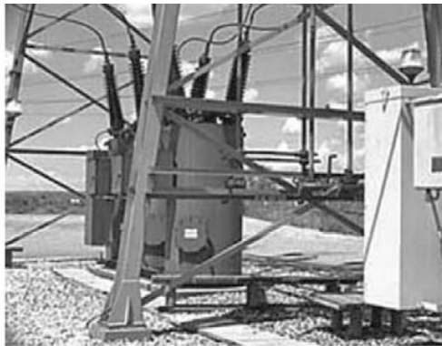
Oil Circuit Breakers in a Circuit
