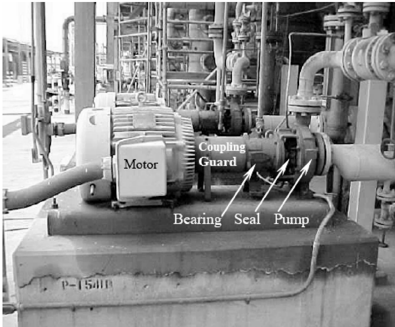
Figure 16.1 A typical industrial pump (courtesy of Dow Chemical Company)
