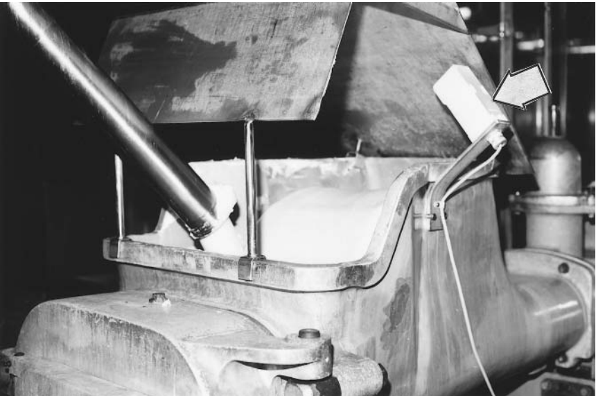
Figure 7 Infrared light sensor ( arrow ) monitors level of butter in hopper and signals computer which controls off/on of delivery pump and an air-operated valve.
