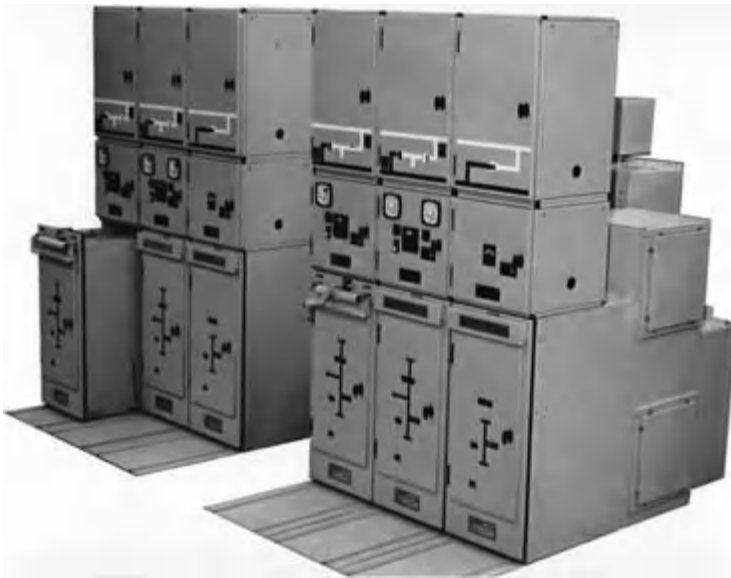
Fig. 2.10 Typical 12 kV metal-clad switchboard using SF 6 circuit-breakers ( Yorkshire Switchgear and Engineering Co. Ltd. ).
