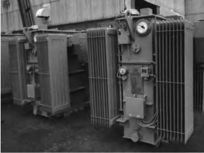
Fig. 13.2 A sealed oil-filled transformer rated at 1600kVA for use in a cement works (Parsons Peebles Distribution Transformers).
