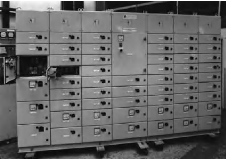
Fig. 2.13 The swing-out design on this l.v. motor control centre gives easy access to the components ( Arcontrol Ltd ).
