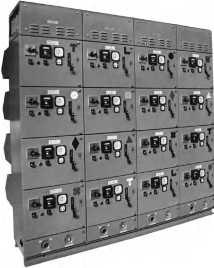
Fig. 2.12 A 400V power station distribution switchboard incorporating air circuit-breakers ( Electro-Mechanical Manufacturing Co. Ltd ).
