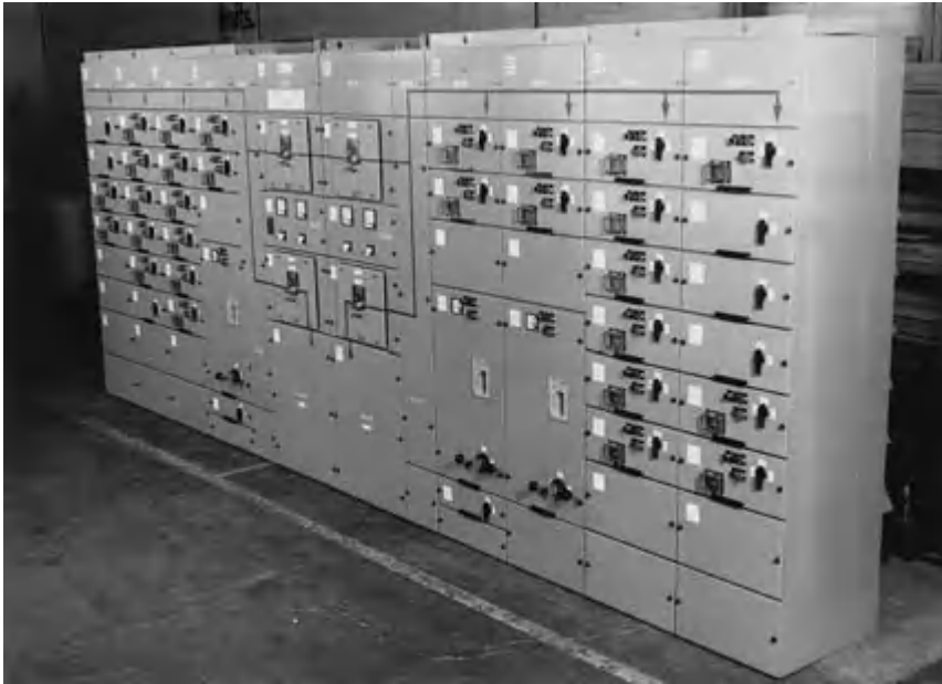
Fig. 17.9 Motor control centres form a compact means of housing many starters.
