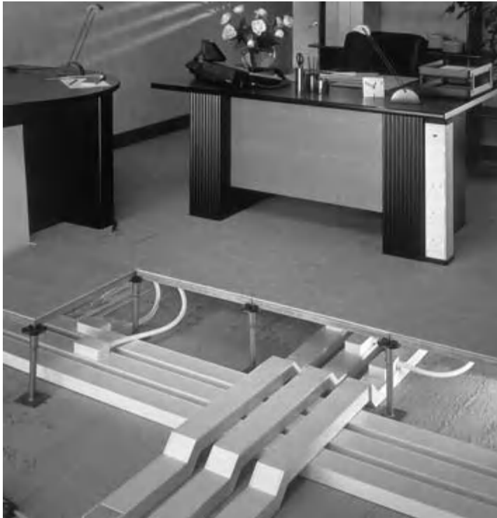
Fig. 4.1 Installed underfloor trunking. Note the segregated circuits.
