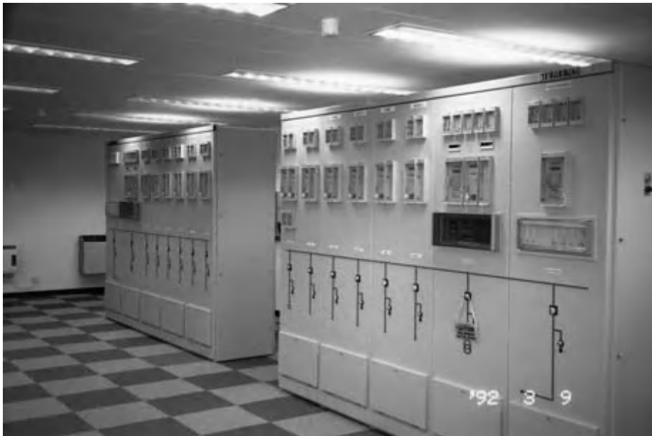
Fig. 2.2 Digital control panel, Jersey ( Siemens plc ).
