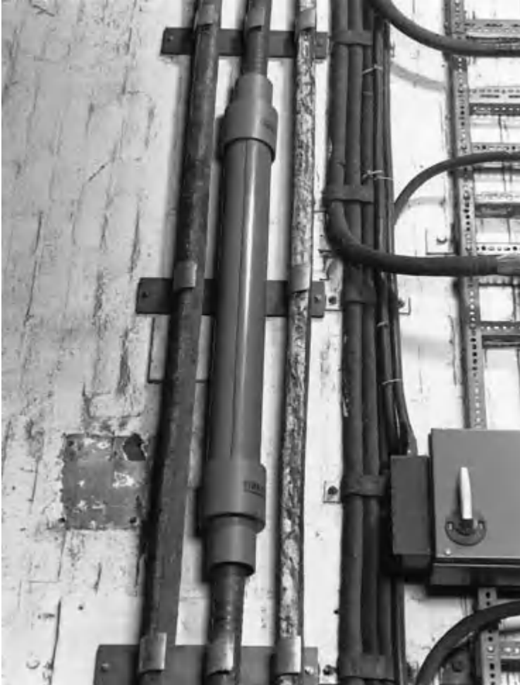
Fig. 19.9 Typical profile of modern straight through joint in 11 kV polymeric-insulated cables ( Pirelli Cables Ltd ).
