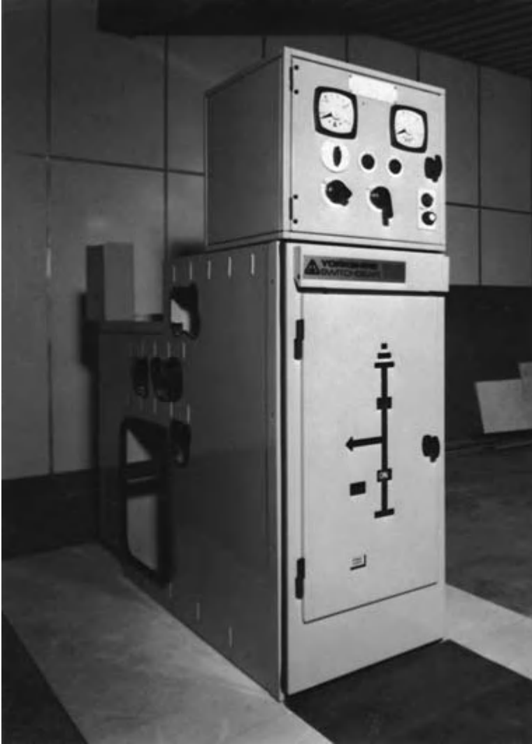
Fig. 14.11 SF 6 switchgear unit with horizontal withdrawal.
