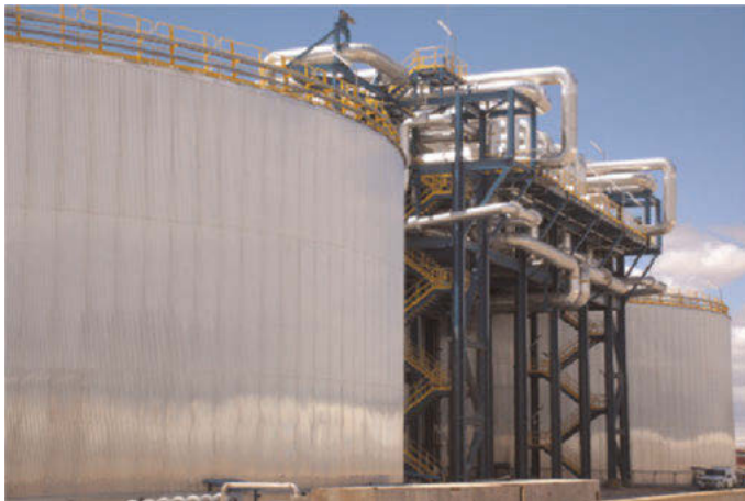
Figure 5.6.3: Example of a 1000 MWh th two-tank molten salt storage system of a concentrating solar power plant in Spain (Source: Andasol 3).
