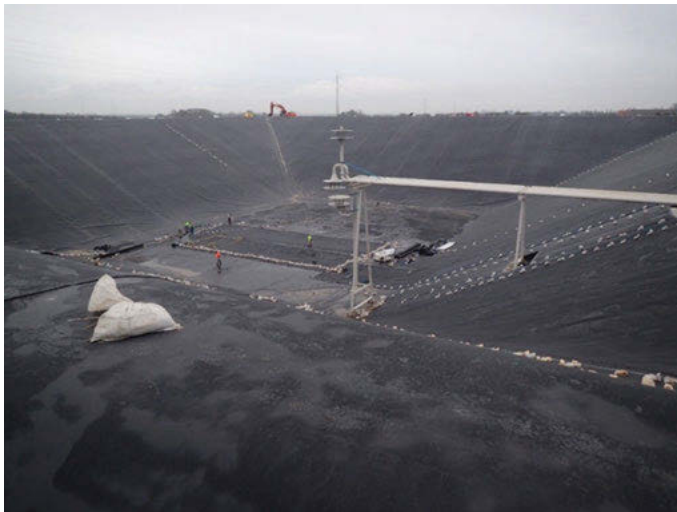
Figure 5.6.1: Pit storage in the construction phase in Toftlund Denmark in 2019. Visible is the plastic liner. The storage is filled with 80000 m 3 water and connected to a heating network (Source Ramboll).
