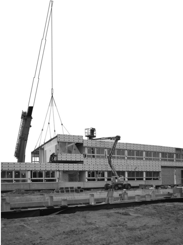
18.5 Construction of the prefabricated steel school building Escola Garigot in Castelldefels, Spain, designed by TAC architects. Courtesy of TAC architects.
