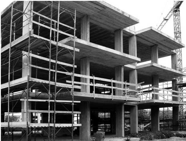
17.2 Construction of an X-Lam building in the European context. Residential building near Verona, Italy, 2010.
