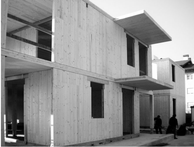
17.1 Construction of a concrete-framed building in the European context. Residential building in Parma, Italy, 2006.
