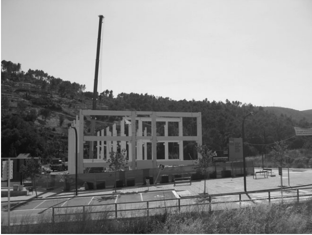
18.3 Assembly of the precast concrete educational edifice Escola Can Coll in Torrelles de Llobregat, Spain, designed by Jordi Canyelles.
