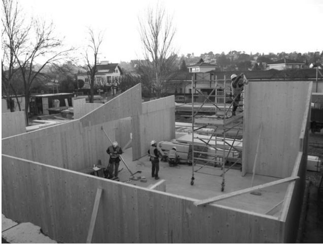
18.7 Assembly of an industrialized wood school edifice Escola Catalunya in Sant Cugat del Vallès, Spain, designed by Xavier Tragant.
