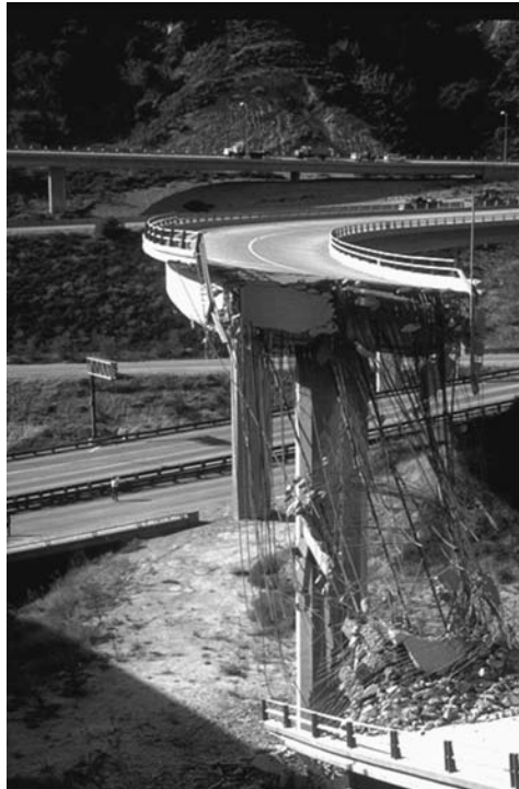
Earthquake-Damaged Bridge (Courtesy of the USGS)
