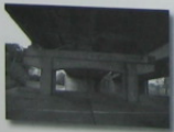
Variable moment-of-inertia concrete piers are sometimes used in the construction of highway bridges.
