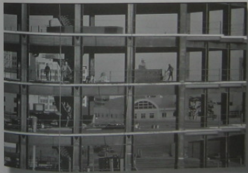
The building framework has rigid connections. A lateral-load analysis can be performed (approximately) by using the cantilever method of analysis.
