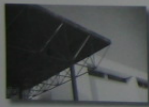
The roof of this pavilion is supported using a system of space trusses.
