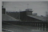
The design of this retaining wall requires estimating the soil pressure acting on it. Also, the gate of the lock will be subjected to hydrostatic pressure that must be considered for its design.
