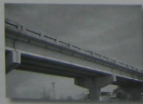
The precast concrete girders are simply supported and are used for this highway bridge. Also, note the tapered beams used to support these girders.
