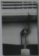
Additional reinforcement, provided by vertical plates called stiffeners , is used over the pin and rocker supports of these bridge girders. Here the reactions will cause large internal shear in the girders and the stiffeners will prevent localized buckling of the girder flanges or web. Also, note the tipping of the rocker support caused by the thermal expansion of the bridge deck.
