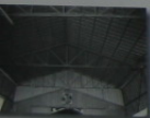
This is an example of a Pratt roof truss. Identify the various members depicted in Fig. 3-2.
