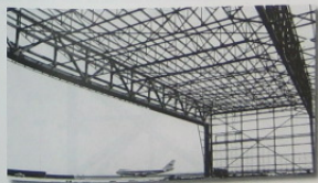
The structural framework of this aircraft hangar is constructed entirely of trusses in order to reduce significantly the weight of the structure. (Courtesy of Bethlehem Steel Corporation)
