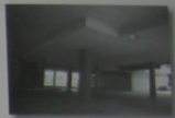
Shown is a typical example of an interior building column. The live load office floor loading it supports can be reduced for purposes of design and analysis.
