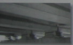
rollers and associated bearing pads are used to support the prestressed concrete girders of a highway bridge.
