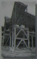
The X-bracing on this frame provides lateral support from wind and vertical support of the floor girders. Notice the use of concrete grout which is applied to insulate the steel to keep it from losing its strength on the event of a fire.
