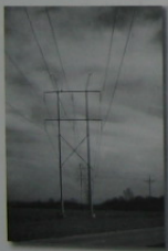
The horizontal members on this power line support frame were designed once the shear and moment within the members were established.
