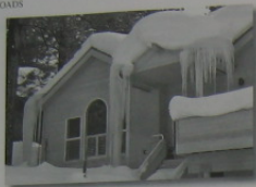
Excessive snow and ice loadings act on this roof.
