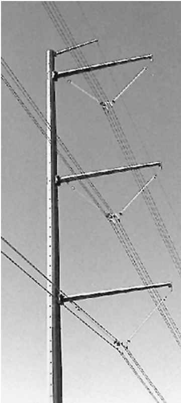
FIGURE 10.1 A 500-kV suspension tower with V string insulators.
