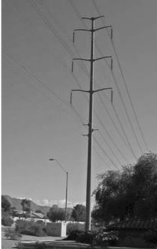
FIGURE 19.4 A 220 kV suspension tower.
