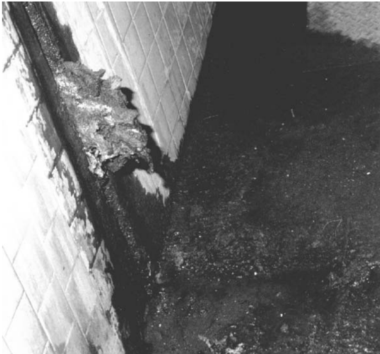
FIGURE 18.11 Liquefaction induced damage to the Webster Street Tube tunnel.
