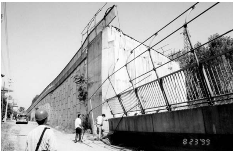
FIGURE 18.73 Mechanically stabilized earth wall continues to support the embankment behind the collapsed Arifiye Overcrossing after the 1999 Kocaeli, Turkey, earthquake.
