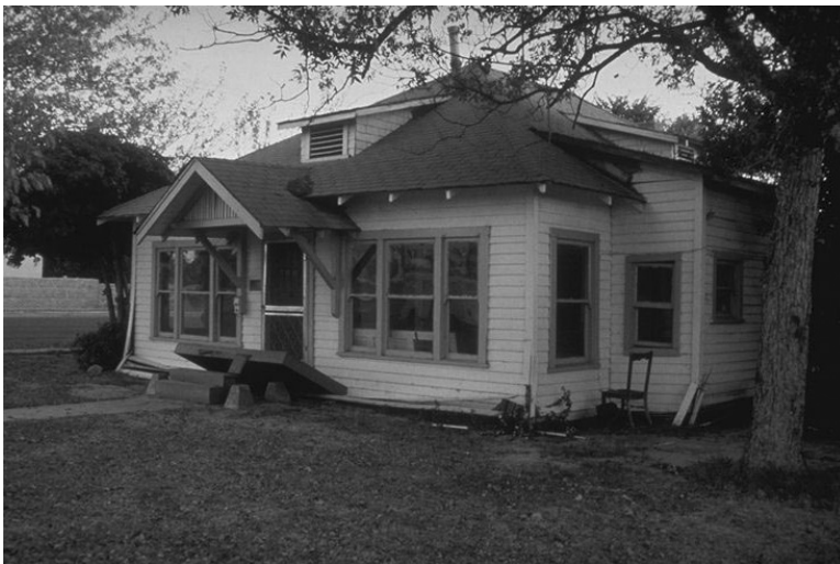
FIGURE 18.34 House that fell from its foundation during the 1971 San Fernando Earthquake. (Photograph courtesy of Steinbrugge Collection, Earthquake Engineering Research Center, University of California, Berkeley.)
