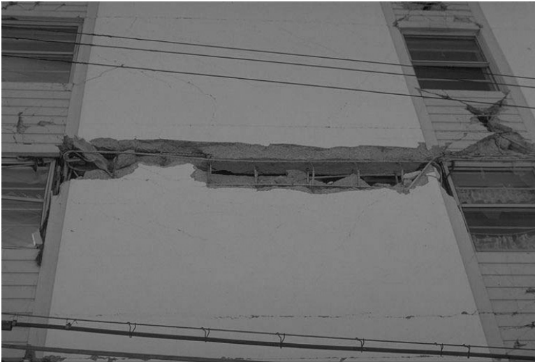
FIGURE 18.49 Damage to north side of Mt. McKinley Apartments. (Photograph by Karl Steinbrugge, Earthquake Engineering Research Center, University of California, Berkeley.)
