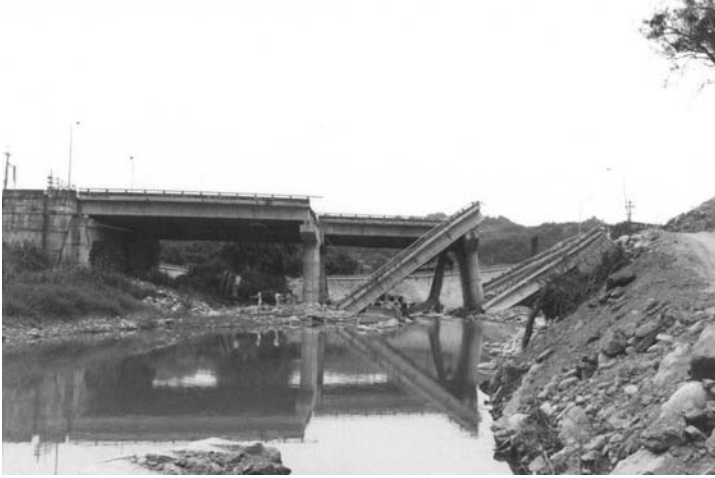
FIGURE 18.19 Collapse of Tsu Wei Bridge due to landslide during the Ji Ji, Taiwan, earthquake.
