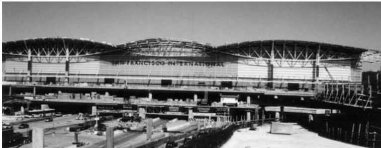
FIGURE 18.77 Construction of the new San Francisco Airport International Terminal. (Photo courtesy of Earthquake Protection Systems Inc.)
