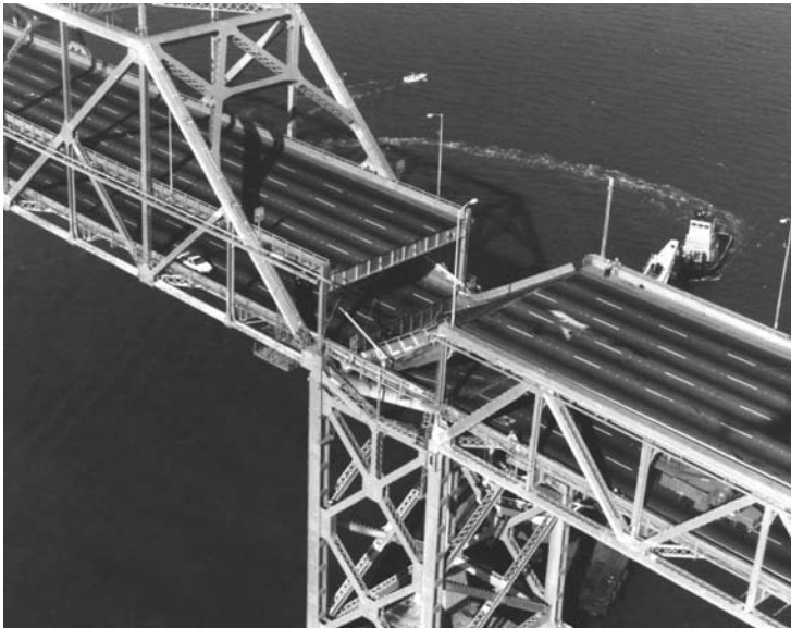
FIGURE 20.1 Collapse of eastern portion of San Francisco–Oakland Bay Bridge in the Loma Prieta Earthquake (courtesy of California Department of Transportation).
