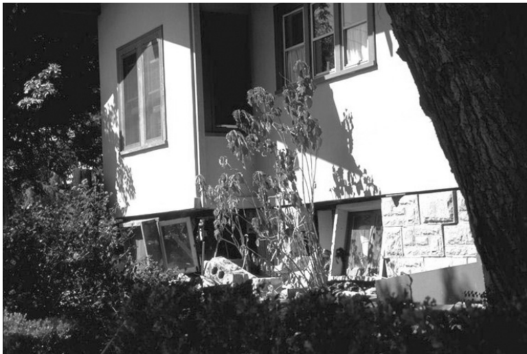
FIGURE 18.32 Failed hollow concrete block foundation during the magnitude 6.0, 1987 Whittier, California, earthquake. (Photo by Karl Steinbrugge. Photo courtesy of Steinbrugge Collection, Earthquake Engineering Research Center, University of California, Berkeley.)
