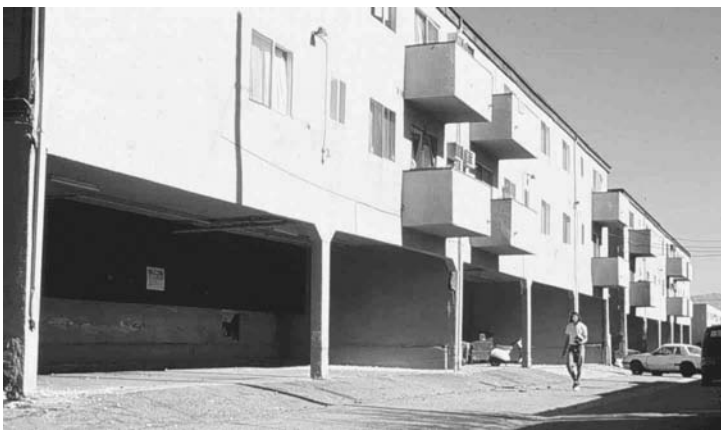
FIGURE 10.7 Typical soft story “tuck-under” parking, with apartments above (courtesy of EQE International).
