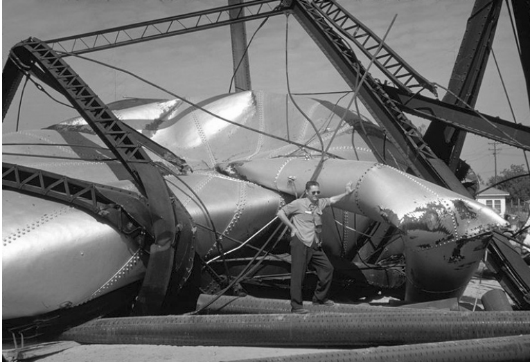
FIGURE 18.62 California Water Service 150,000-gal tank on six legs; the typical failure of tanks is upside down, with riser on top (Bakersfield, California, photo by Karl V. Steinbrugge, Steinbrugge Collection, slide/image No. S64, photo date July 25, 1952, Kern County, California, earthquake, July 21, 1952, magnitude 7.69; courtesy of Steinbrugge Collection, Earthquake Engineering Research Center, University of California, Berkeley).
