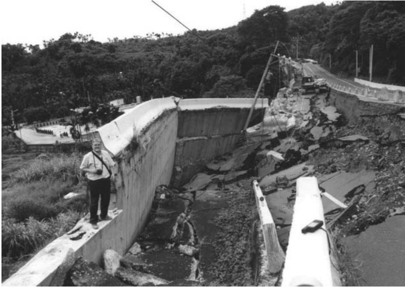
FIGURE 18.13 Gravity retaining wall pushed outward by landslide.
