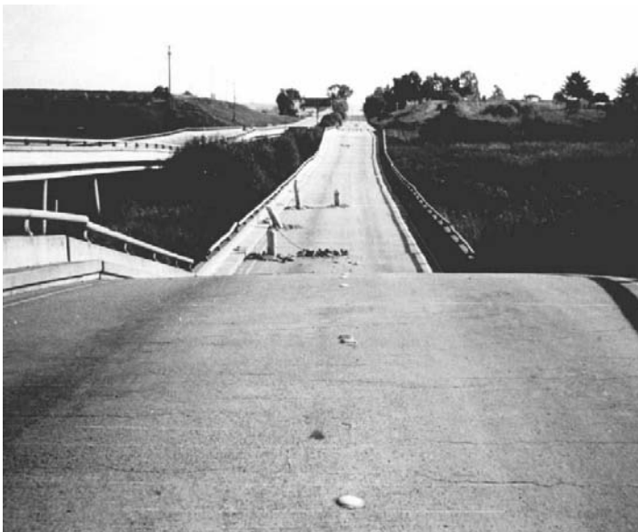
FIGURE 18.26 Piles penetrating bridge deck.
