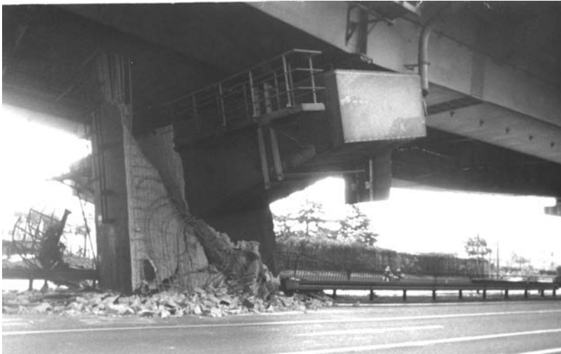
FIGURE 18.51 Shear failure of Pier 150 on Kobe Route 3.
