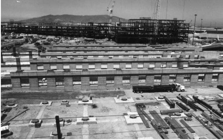
FIGURE 18.78 Layout of foundations and friction pendulum devices for the new San Francisco Airport International Terminal. (Photo courtesy of Earthquake Protection Systems Inc.)
