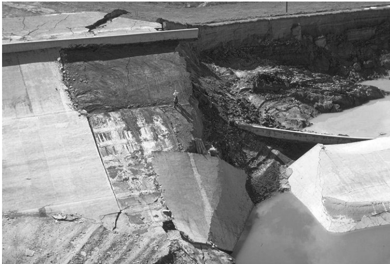
FIGURE 18.22 Closer view of damage to the Lower San Fernando Dam. (Photograph courtesy of Steinbrugge Collection, Earthquake Engineering Research Center, University of California, Berkeley.)
