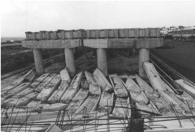
FIGURE 18.63 Collapsed precast, prestressed “I” girders during construction of new expressway in Taiwan due to the 1999 Ji Ji, Taiwan, earthquake.
