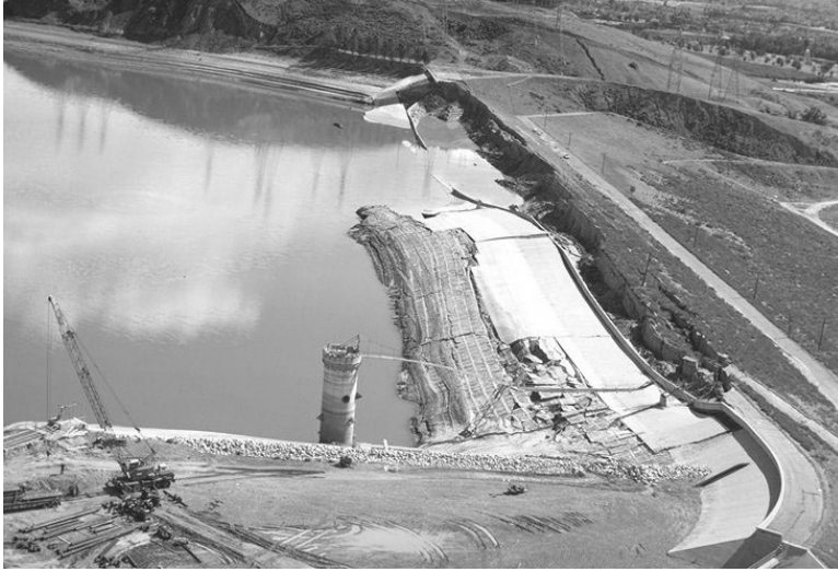
FIGURE 18.21 Damage to the Lower San Fernando Dam. (Photograph courtesy of Steinbrugge Collection, Earthquake Engineering Research Center, University of California, Berkeley.)
