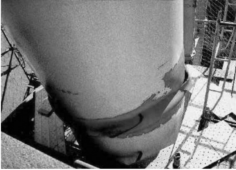
FIGURE 18.55 Torn buckle of steel column on Route 3 after the 1995 Kobe Earthquake. (Photo courtesy of Hanshin Expressway Public Corporation.)
