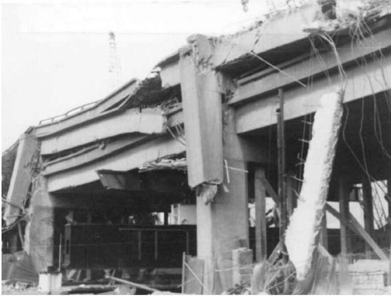
FIGURE 18.28 Damage to Cypress Street Viaduct.
