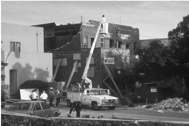
FIGURE 18.61 Rear view of damaged unreinforced masonry (URM) building facing Pacific Garden Mall, Santa Cruz Area, California. (Photo by James R. Blacklock, Loma Prieta Collection, Earthquake Engineering Research Center, University of California, Berkeley.)
