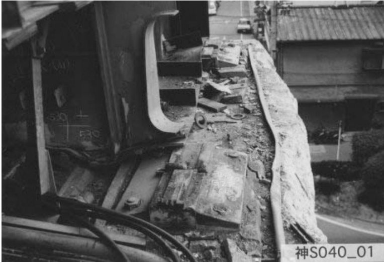
FIGURE 18.58 Broken bearings at Pier 40. (Photo courtesy of Hanshin Expressway Public Corporation.)
