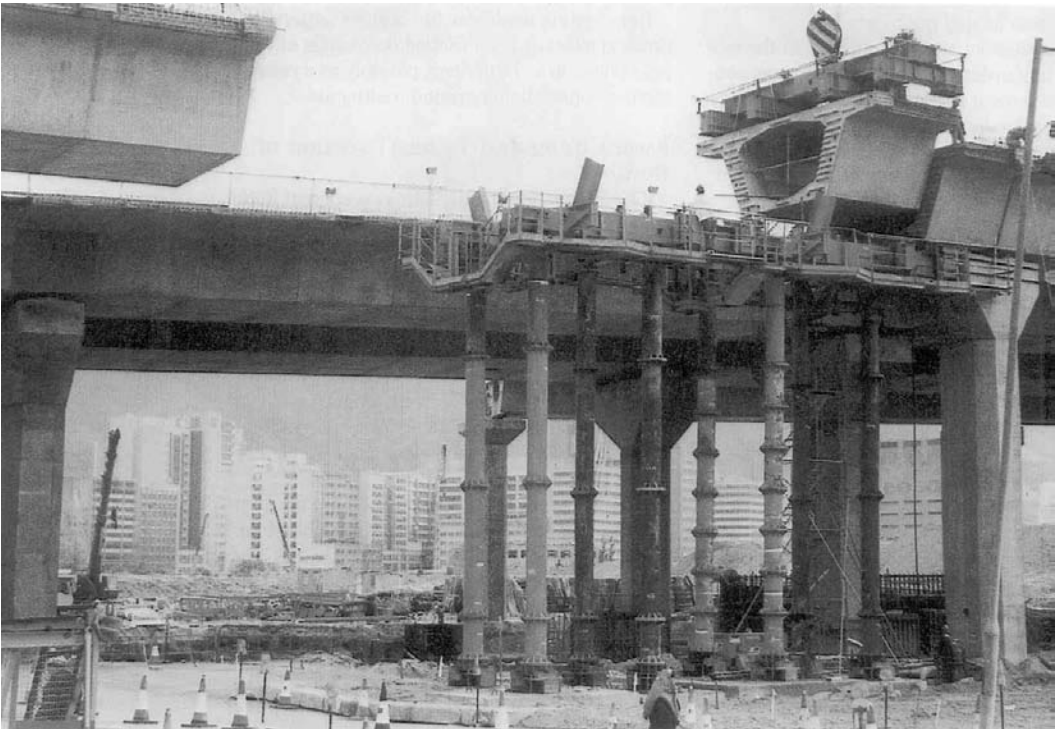
PHOTO 8.8 West Kowloon Expressway Viaduct, Hong Kong, during construction, comprising 4.2 km dual three-lane causeway connecting Western Harbor Crossing to new airport (courtesy Institution of Civil Engineers, London, and [5]).
