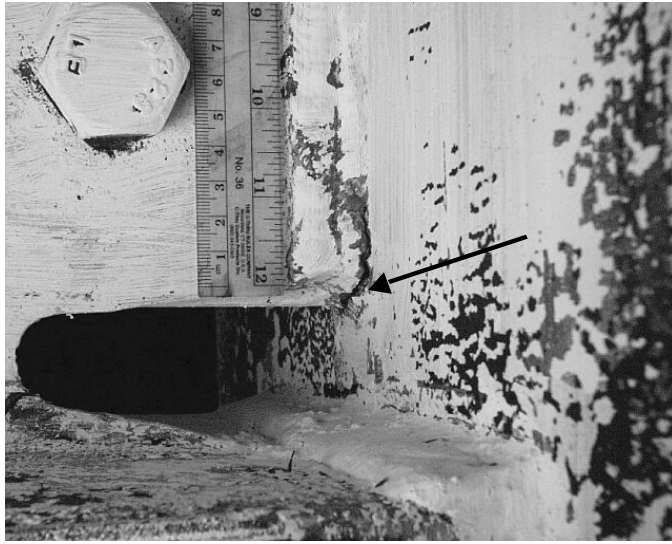
FIGURE 34.8 Low-cycle fatigue crack developing at the end of the beam web to column flange weld in a moment-frame connection.
