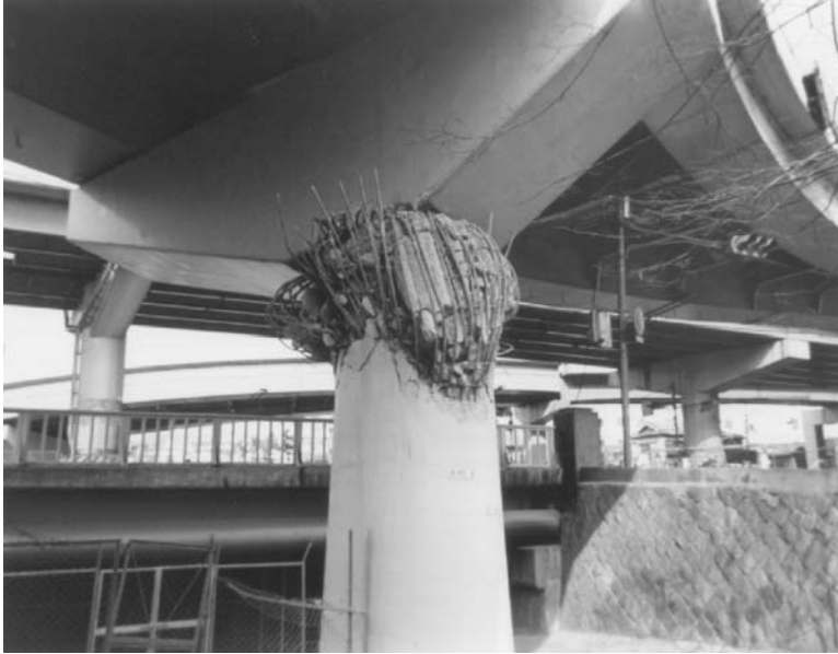
FIGURE 18.46 Column damage to the Minatogawa interchange during the Kobe Earthquake.
