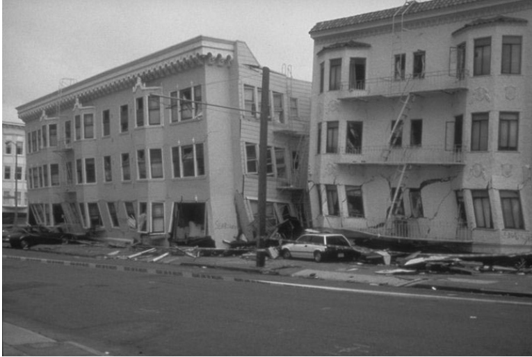
FIGURE 18.37 Soft story collapse in San Francisco during the 1989 Loma Prieta Earthquake. (Photo courtesy of the USGS; The Loma Prieta, USGS, 1998.)
