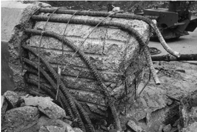
FIGURE 18.36 Failure of column to footing connection.
