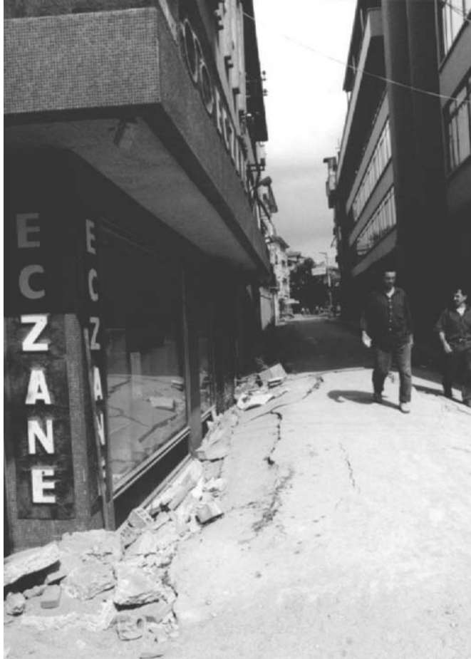
FIGURE 18.6 Settlement of building due to loss of bearing during the 1999 Kocaeli Earthquake.
