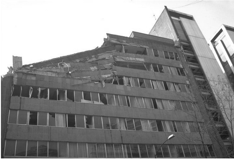
FIGURE 18.31 Damaged 10-story building between the Plaza de la Constitución and Zona Rosa in Mexico City. (Photo by Karl Steinbrugge, from the EERC NISEE Photo Library.)
