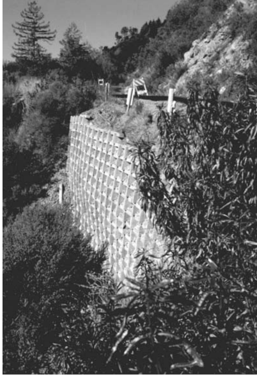
FIGURE 18.74 Crib wall continues to support steeply sloping soil in Santa Cruz after the 1989 Loma Prieta Earthquake. (Photo courtesy of EERI.)
