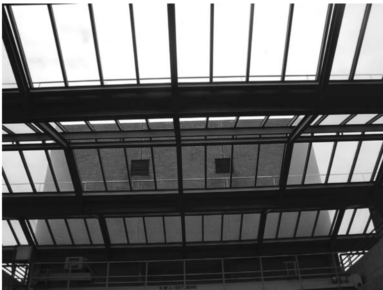
FIGURE 29.8 Broken glass panel due to thermal stress.
