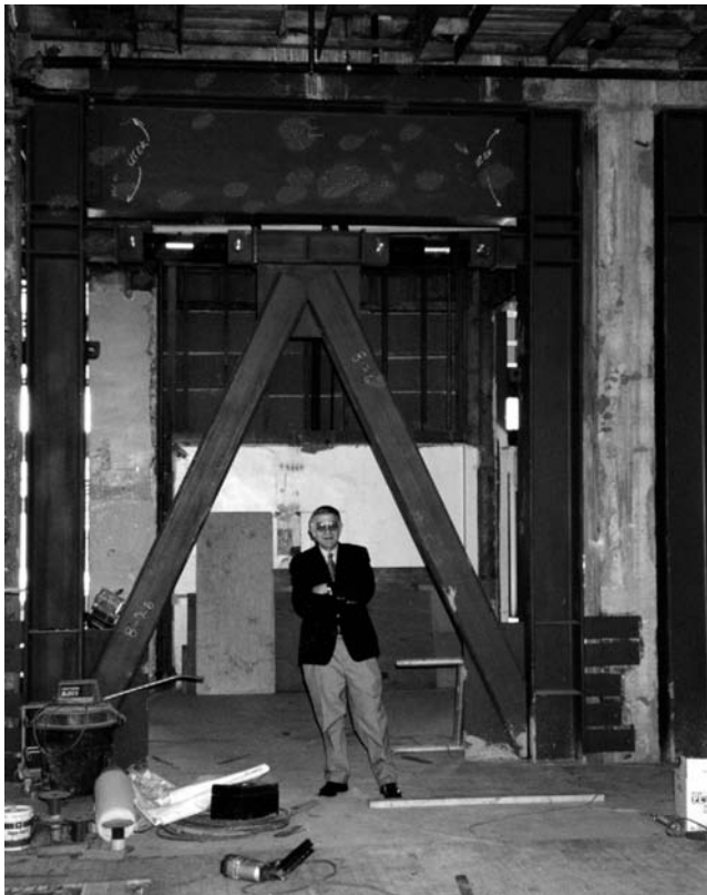
FIGURE 18.83 The steel frames included fluid viscous dampers to reduce the story drift. (Photo courtesy of Marr-Shaffer & Miyamoto, Structural Engineers.)
