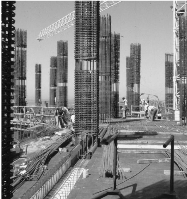
PHOTO 7.2 Installation of reinforcing bars in the Pacific Park Plaza building (courtesy of Mr. James Tai, T.Y. International, San Francisco).
