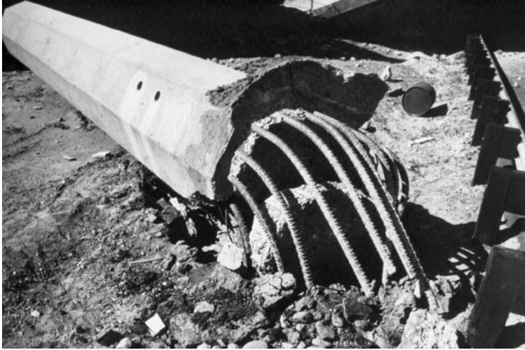
FIGURE 18.35 Failure of column to pile shaft connection.
