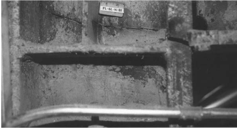
FIGURE 18.60 Steel moment-resisting frame connection after the 1994 Northridge Earthquake. (Photo courtesy of EQE International; EQE, EQE Int. Rev. , Fall, 1–6, 1994.)
