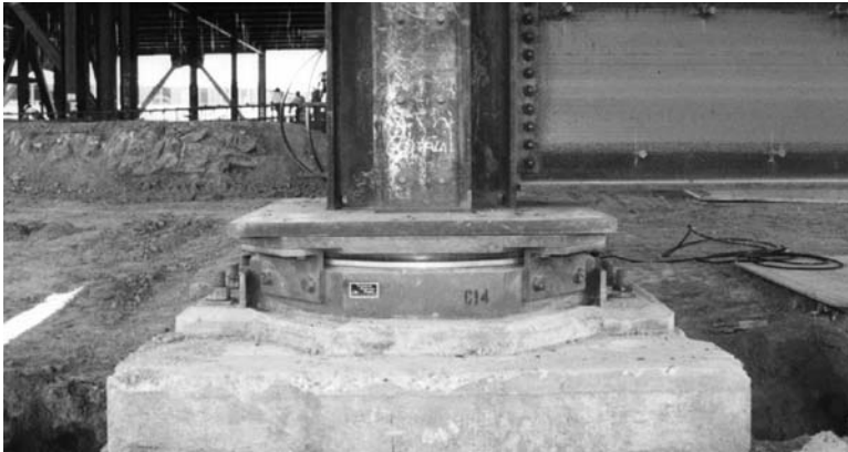
FIGURE 18.79 One of the 267 friction pendulum devices for the new San Francisco Airport International Terminal. (Photo courtesy of Earthquake Protection Systems Inc.)
