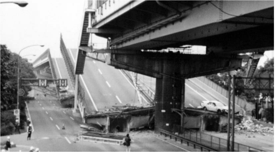
FIGURE 18.56 Superstructure collapse at Spans 40 and 41 on Kobe Route 3.
