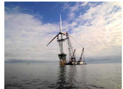
Figure 10.8. Construction of the Beatrice demonstrator deep offshore windfarm. Photos kindly provided by Talisman Energy (UK) Limited.
