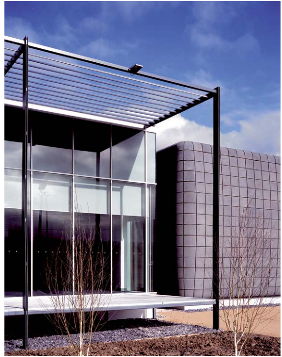
Fig. 3.19 Reconstructed stone cladding – Experian Data Centre, Nottingham. Photograph: Courtesy of Trent Concrete Ltd
