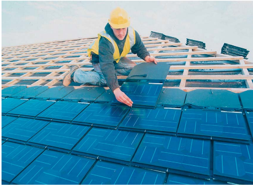
Fig. 14.3 Photovoltaic slates. Photograph: solarcentury.com
