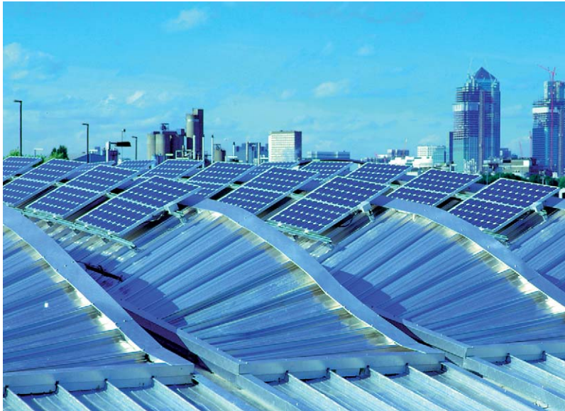
Fig. 14.2 Photovoltaic array. Photograph: solarcentury.com
