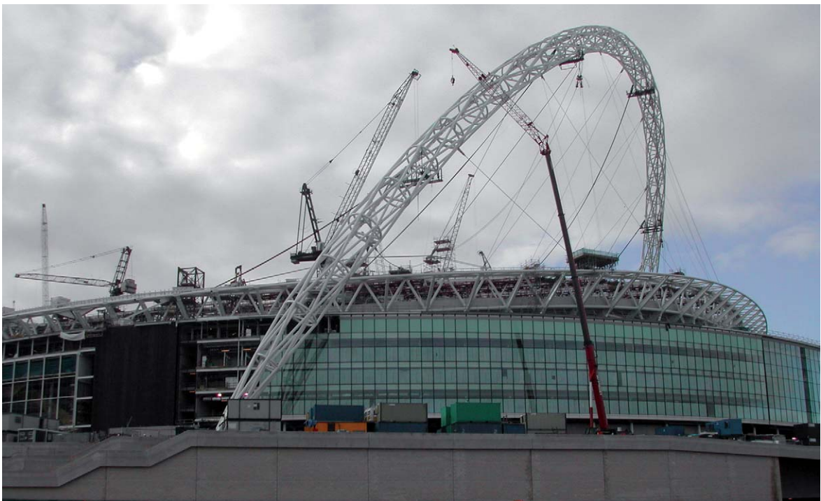
Fig. 5.9 Structural steelwork – Wembley Stadium, London. Architects: Foster and Partners. Photograph: Arthur Lyons
