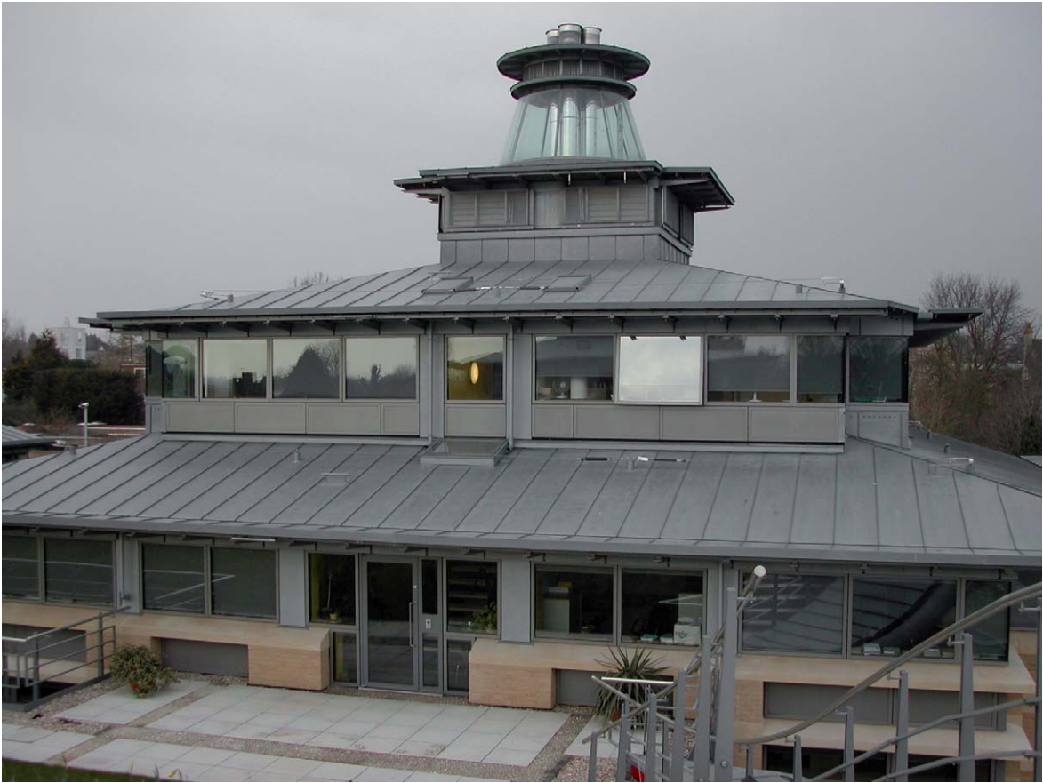
Fig. 5.28 Zinc alloy roofing – Centre for Mathematical Sciences, University of Cambridge. Architects: Edward Cullinan Architects. Photograph: Arthur Lyons
