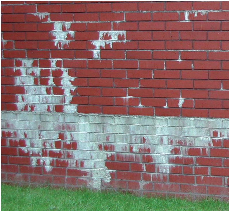
Fig. 1.10 Lime leaching on brickwork
