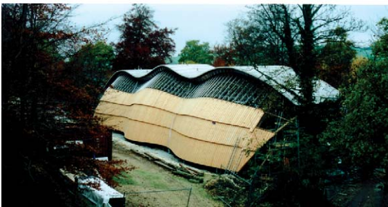
Fig. 4.15 Gridshell construction – Weald and Downland Open-Air Museum. Architects: Edward Cullinan Architects. Photograph: Courtesy of Edward Cullinan Architects
