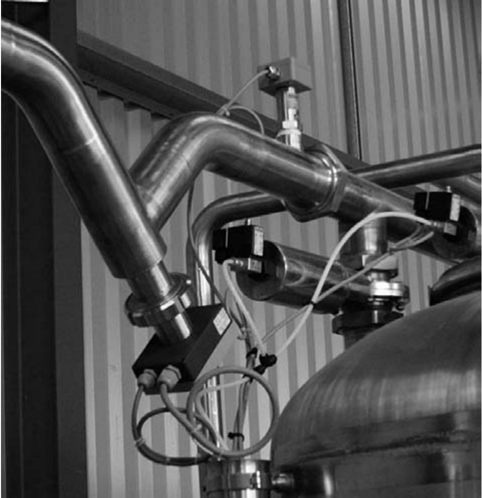
Fig. 7.8 Typical conductivity/temperature probe and flow switch.
