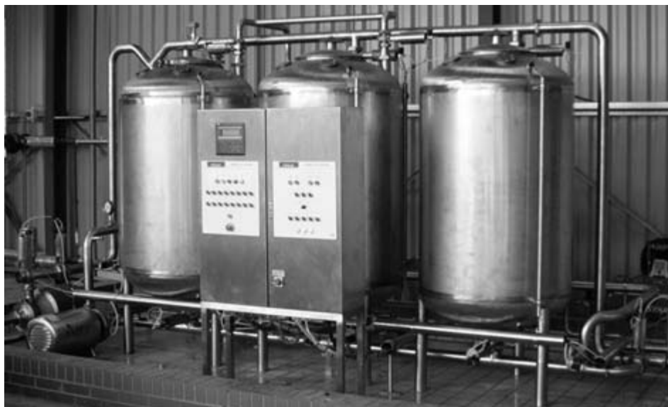
Fig. 7.1 A general view of the CIP cleaning system.
