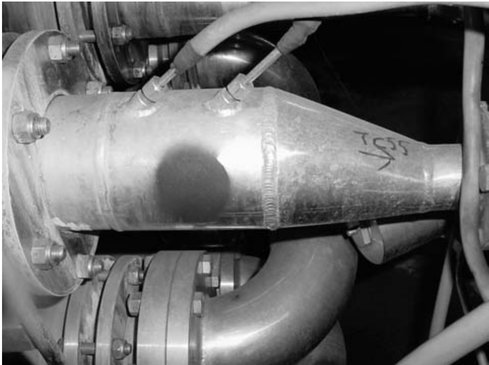
Fig. 8.2 Double Pt100 thermocouple positioned at a tube outlet. Reproduced by permission of Unilever R&D, Bedford, UK.
